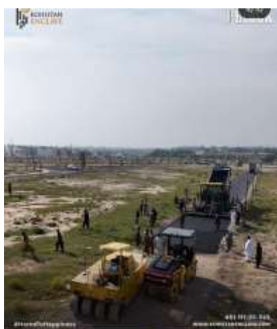
kohistanenclave With every step forward, Kohistan Enclave reinforces its reputation for quality development. Asphalt work in progress at I Block, Precinct 5 ensuring commitment to delivering infrastructure that reflects precision, quality, and long-term value for our residents and investors. less
